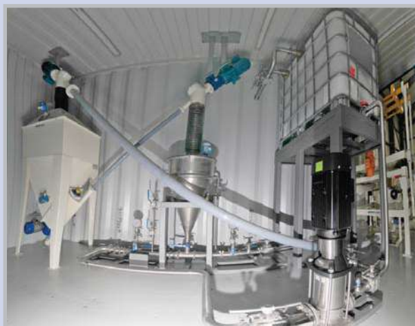
Water treatment system inside an ISO container
