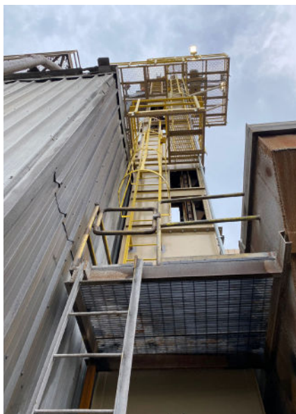
Bucket elevator with service platform, ladder with safety cage, and explosion vent panels (not yet installed)
