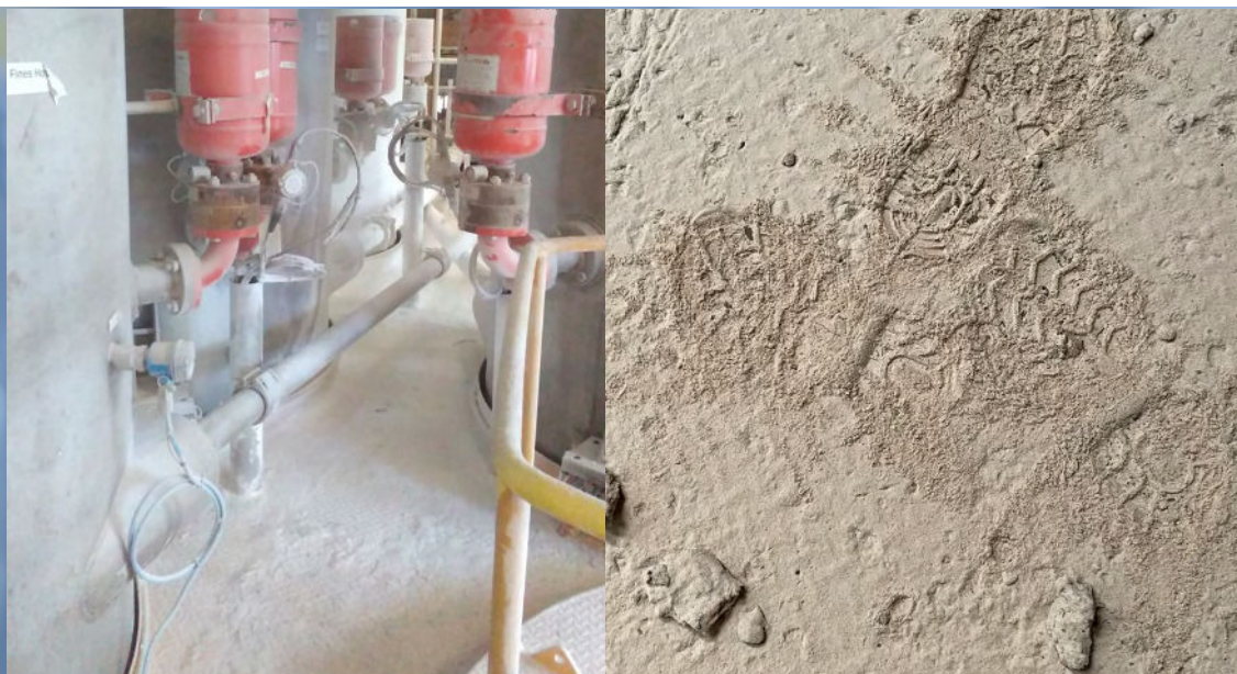
Figure 1 – Dust accumulations. External Zone 22 may be required – Housekeeping improvements would be preferable!
