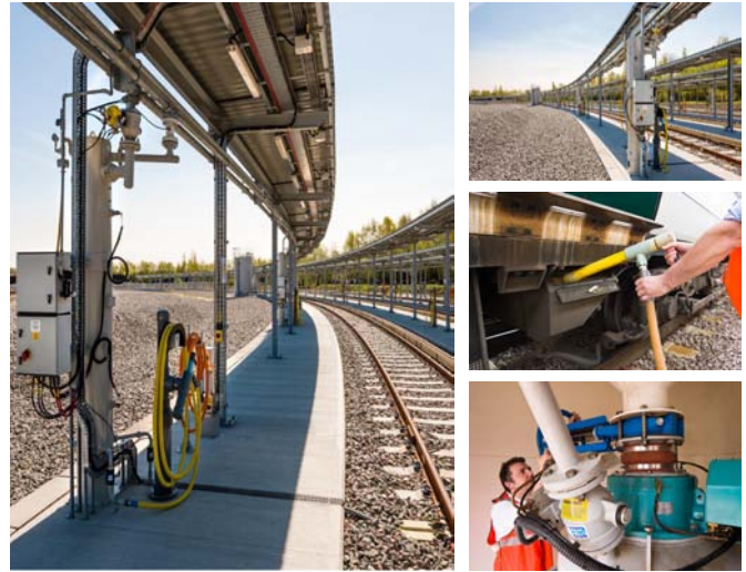
Selhurst Field sidings Sand Filling Station
