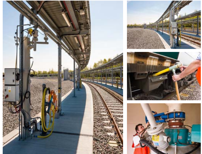
Selhurst Field sidings Sand Filling Station
