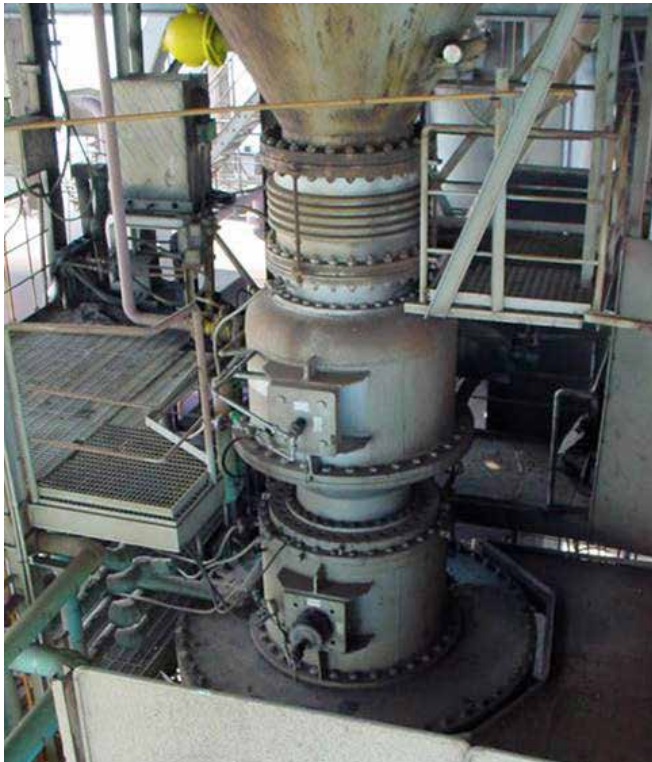
Clyde Process Clam and Ball Valves controlling Gasifier lock hoppers
