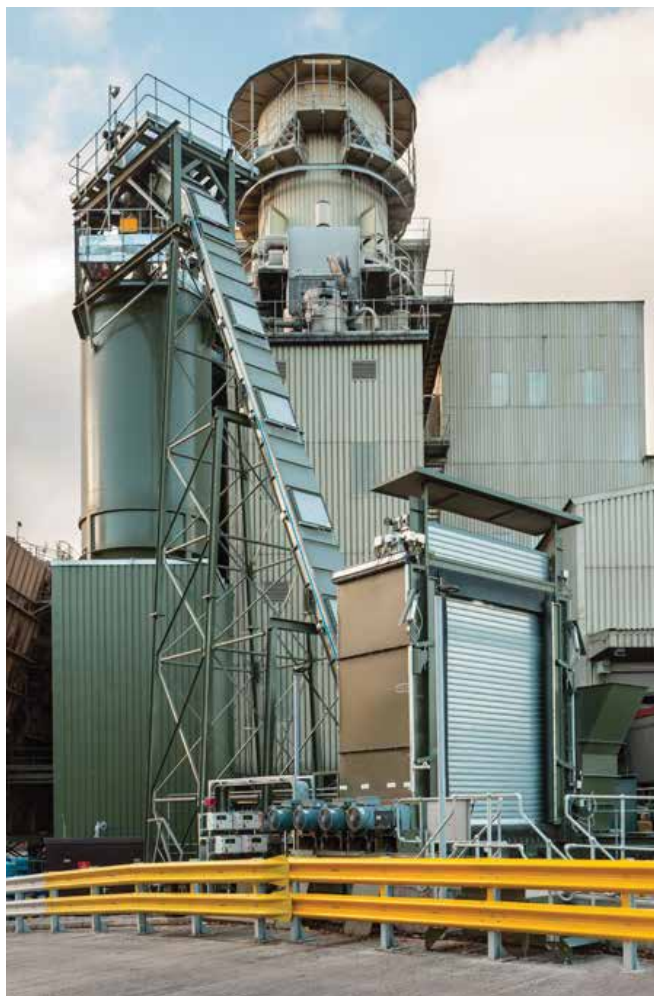
PSP material receiving station, conveyor and storage silo
