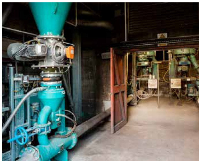
MULTICOR® K Feeder for PSP material feeding into the same pipeline as the existing coal feeders
