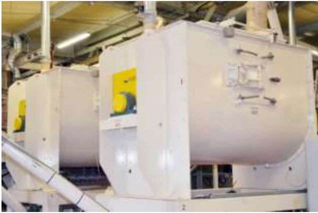
Figure 2 John R Boone HHBM mixers at Exwold Chemicals
